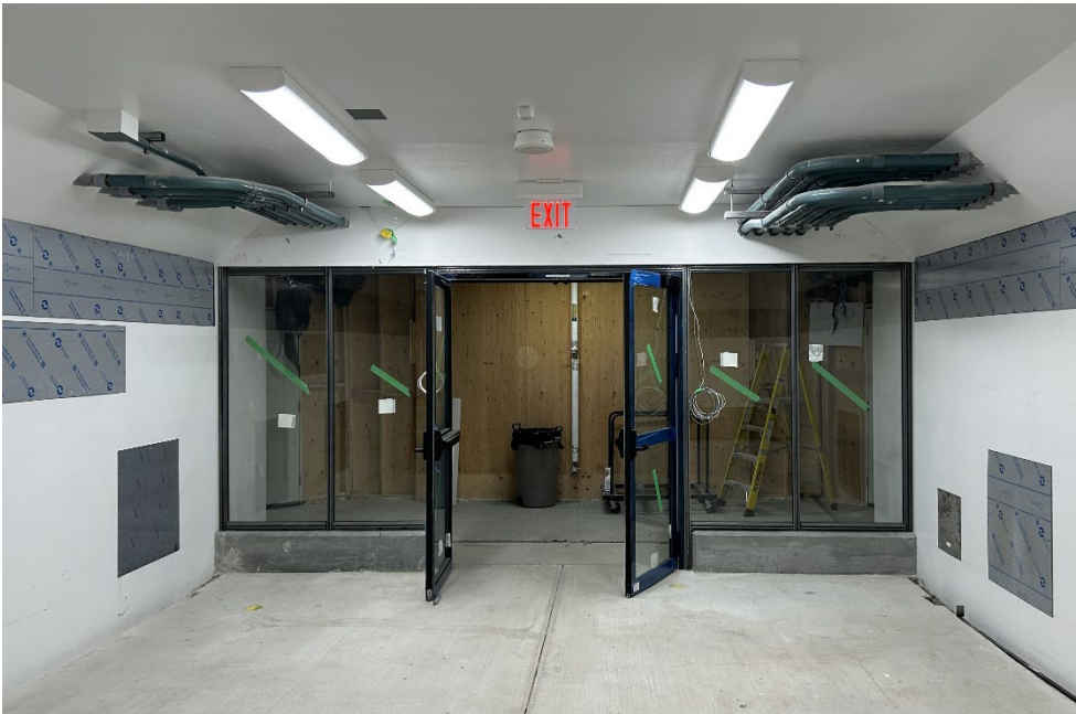
Figure 1: Fire rated partition and door
