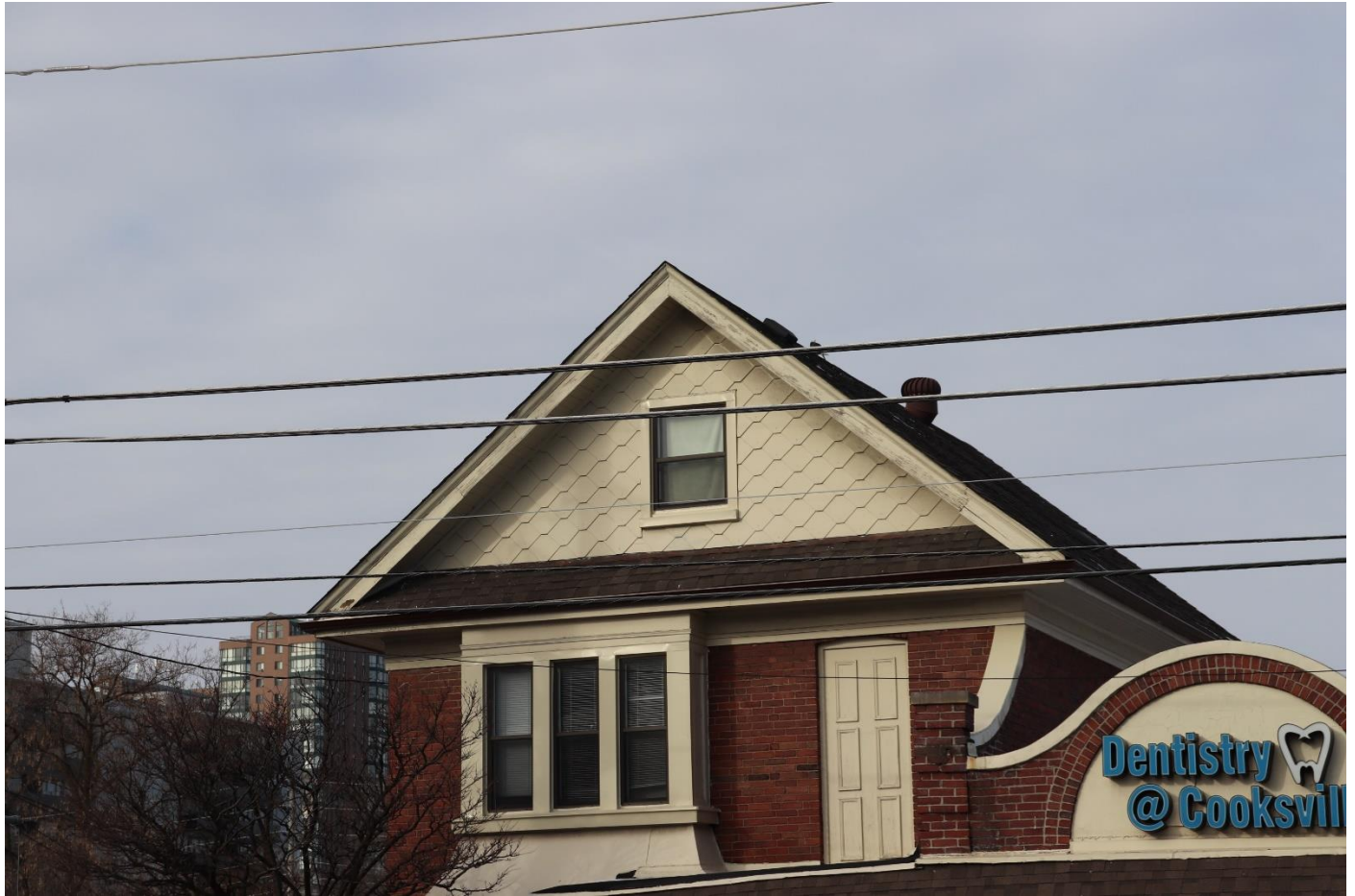
Photograph 2: Close-up of the attic gable and window with imbricated, fish scale style wood shingles (AECOM, 2021)
