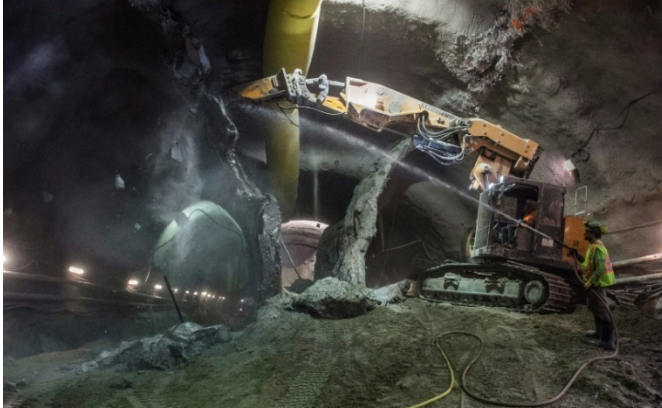
A behind-the-scenes look at tunneling taking place underneath Avenue Station on the Crosstown.
