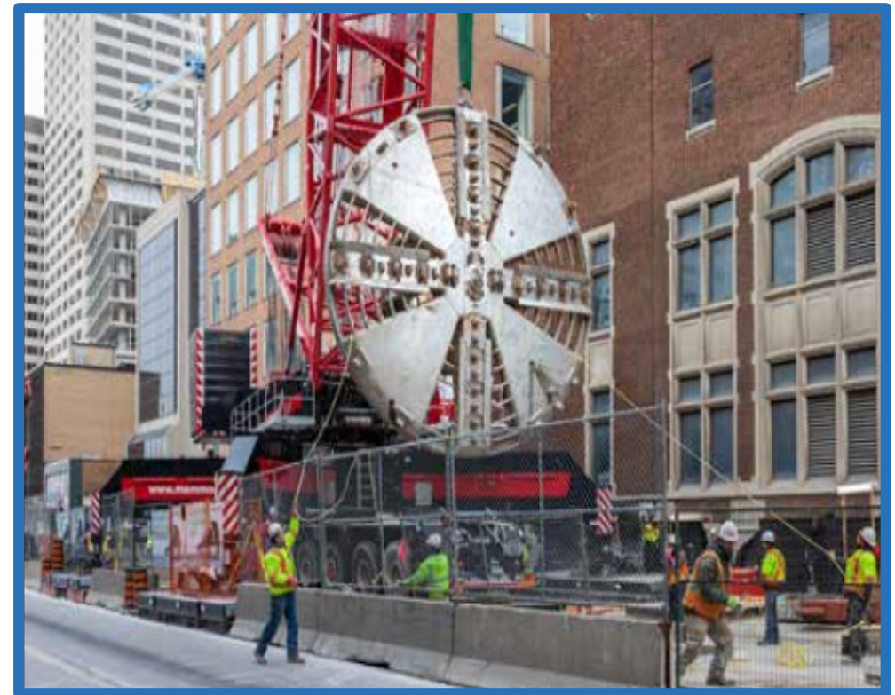
Eglinton Crosstown LRT tunnel boring machine extraction near Eglinton Ave. and Yonge St.
