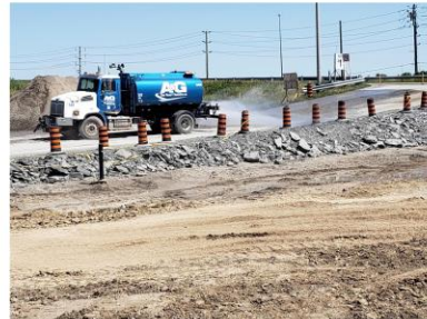
Example of trucks spraying water as part of dust control mitigation for the surrounding community. Source: Metrolinx, 2020.
