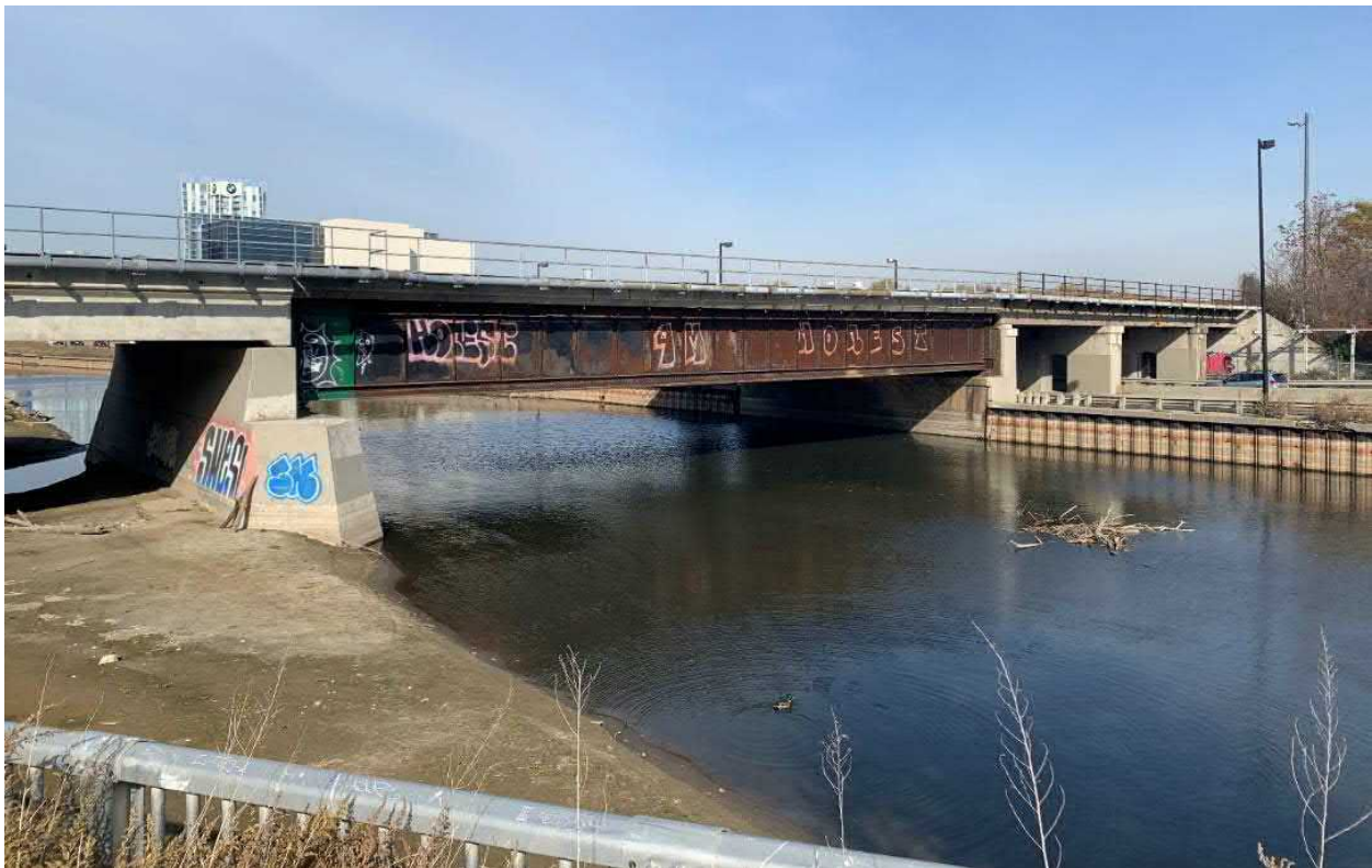
Image 1: View of the south side of the Lakeshore East rail bridge within the Lower Don Bridge and Don Yard Study Area (Photograph taken by AECOM in 2020)
