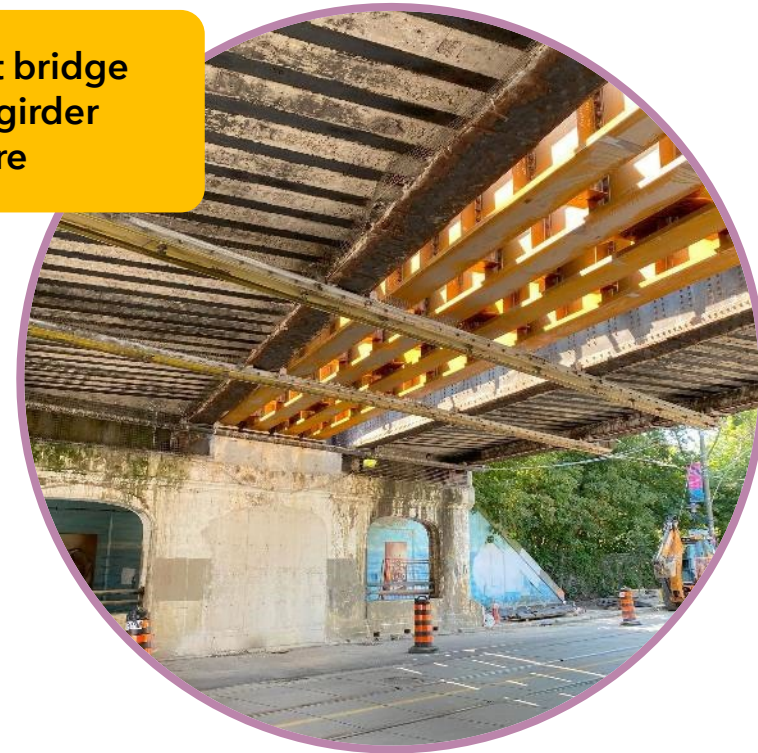
Dump trucks will be used to remove demolished materials from the bridge
