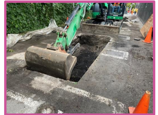
Excavating a Stage 2 trench on a City of Toronto bike path, facing west
