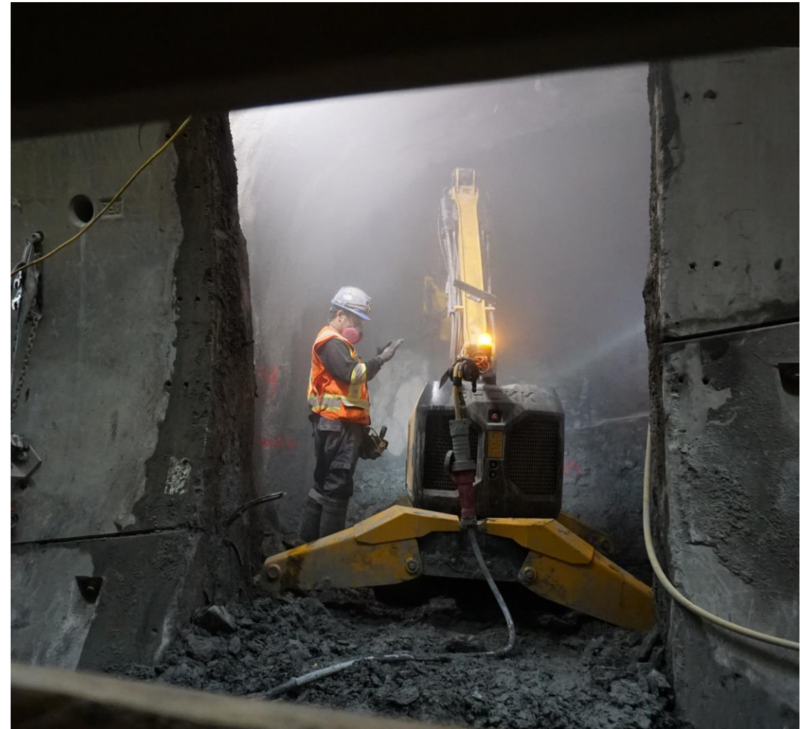
Photo Credit: Yusuf Soliman, Tunnel / Geotechnical Engineer from Dr. G. Sauer & Partners Corp
