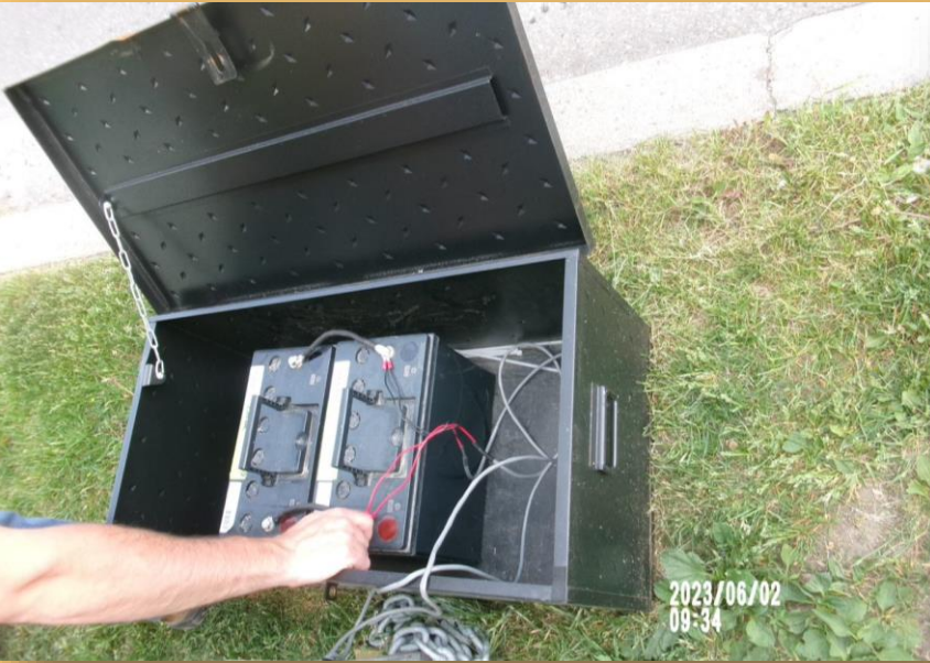
Noise and vibration monitor in front of TPSS
