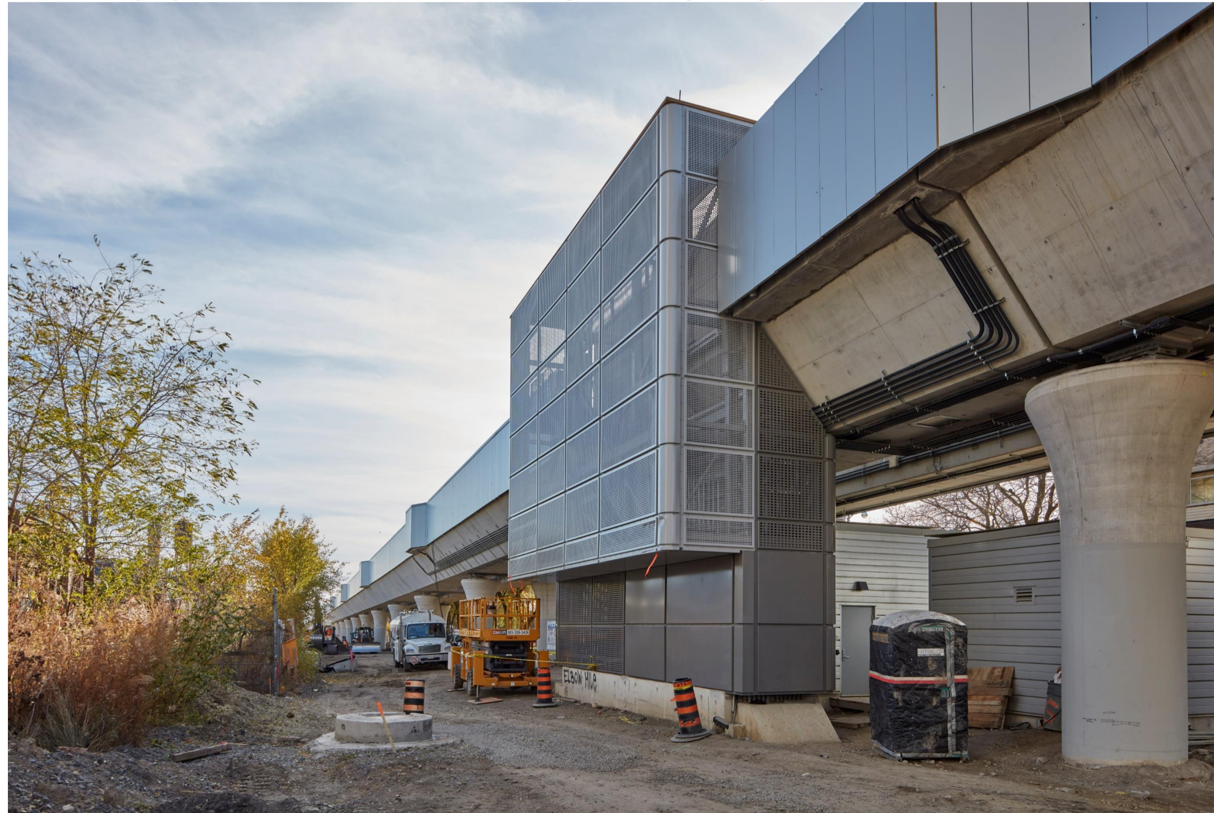
Electrical and Communications Rooms and Emergency Egress Stairway.
