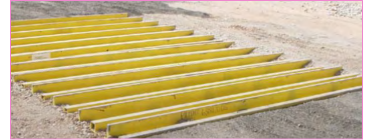
Shaker Rack, for truck wheel cleaning
