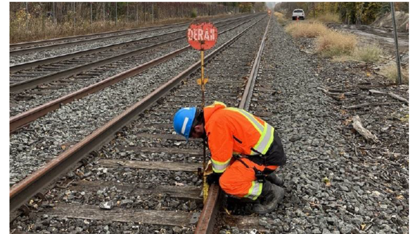
A&B rail installing a portable derailed rail in accordance with CROR-841 protection.
