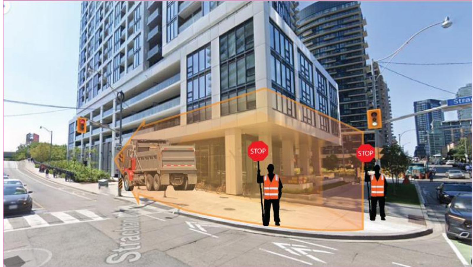
Approximate location and set up of the trucking access point, via Strachan Avenue. NOTE: This plan is in development, including review of safety measures and pedestrian accommodation.
