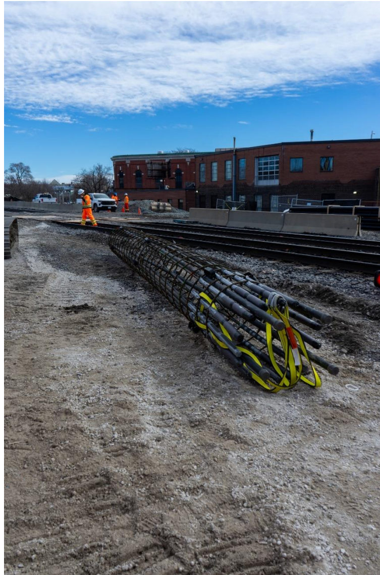
Steel rebar structure that will serve as foundation when filled with concrete
