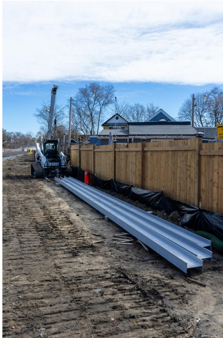
Steel piles waiting to be installed into the ground. These will support noise barriers.
