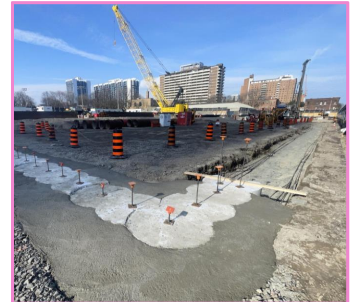
Typical example of guide wall installation to properly align the secant piles
