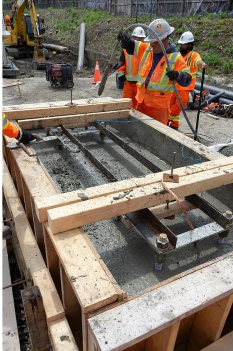
A concrete vibrator is inserted during the pour to liquify it and help it settle evenly
