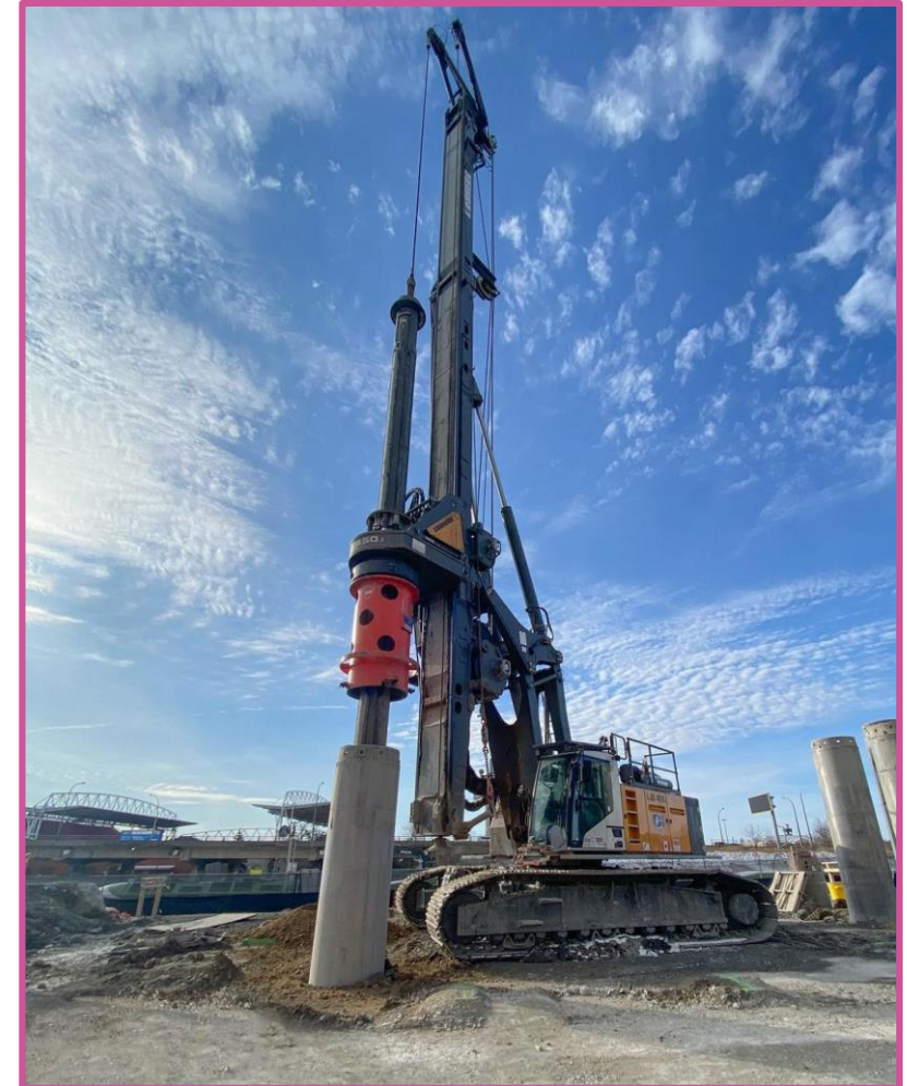
A drill rig machine used in Ontario Line project used for piling.
