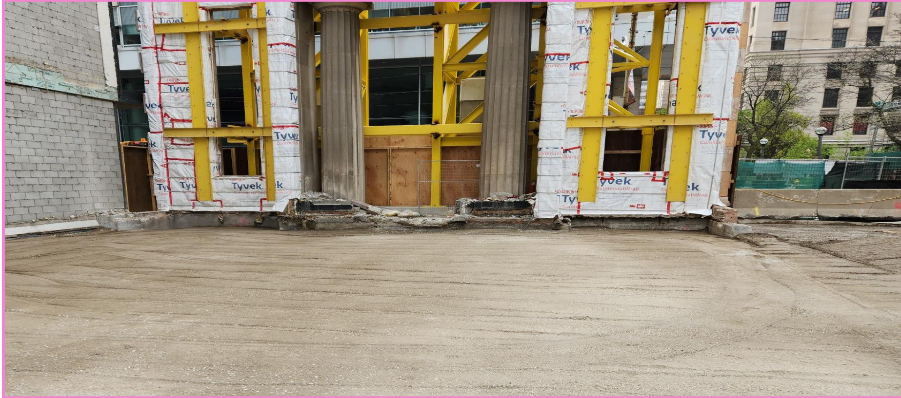
View from inside the future South station entrance after crews completed backfilling the ground to level it prior to piling.
