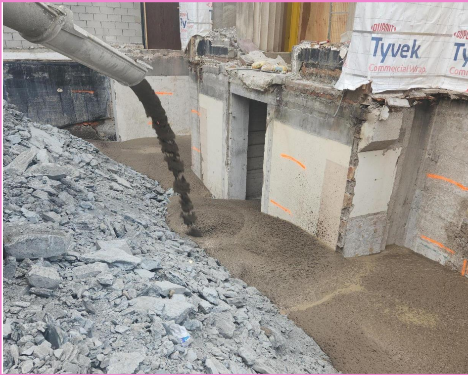
View of work to backfill the basement at the future South station entrance with shale. This work is done to provide a solid and stable base.
