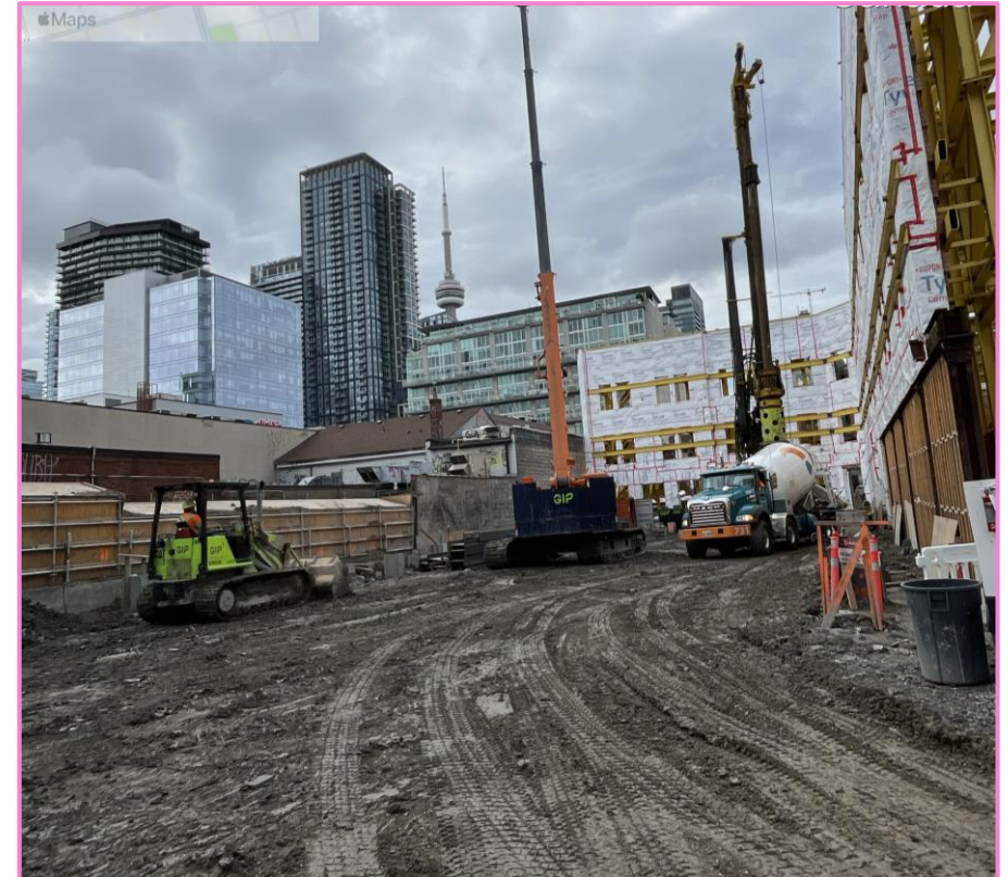
View of ongoing works at the future North station site as of May 25, 2024
