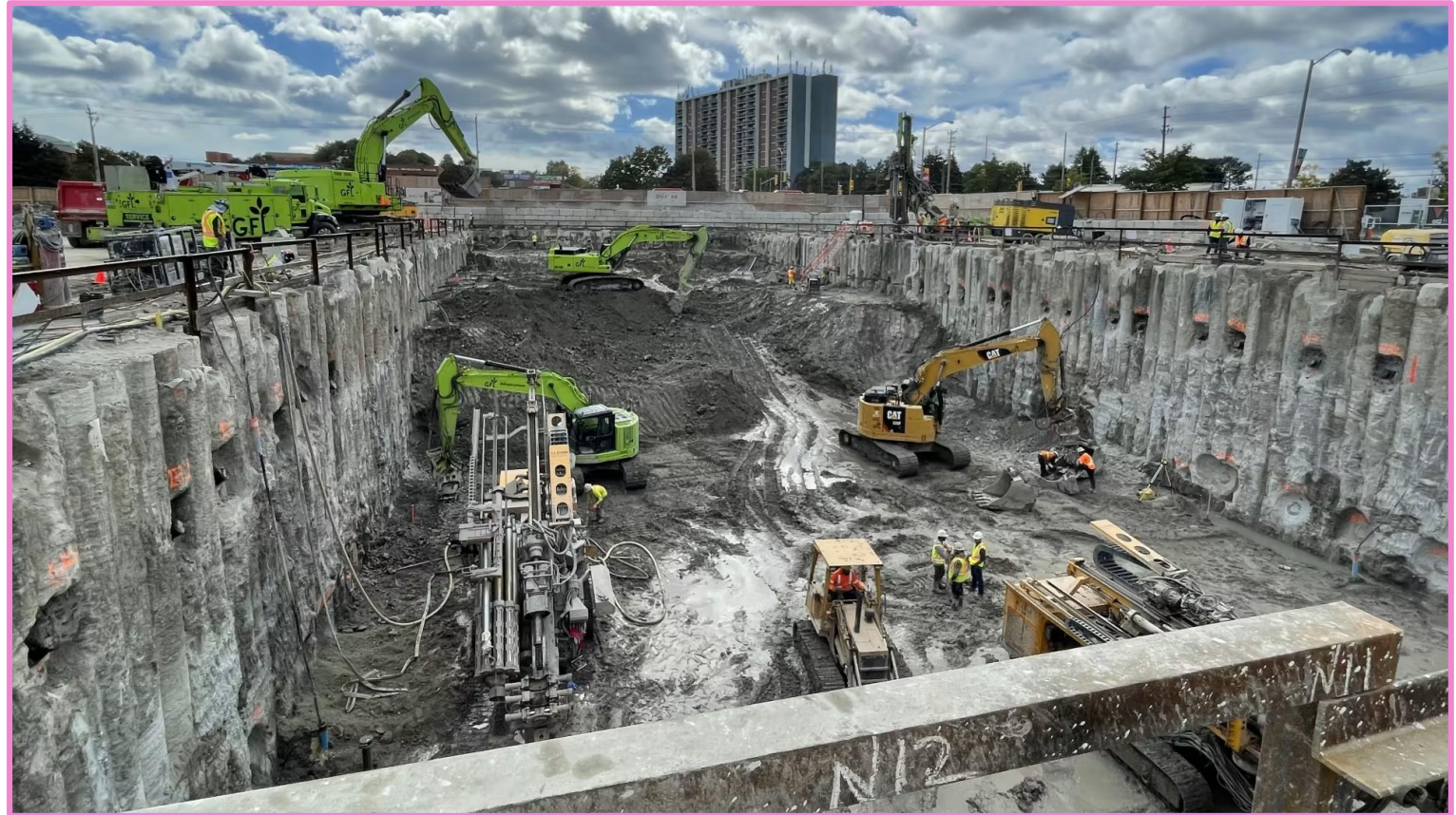
Excavators and other heavy machinery are digging deep to build the launch shaft for the tunnel boring machine. (Metrolinx image)
