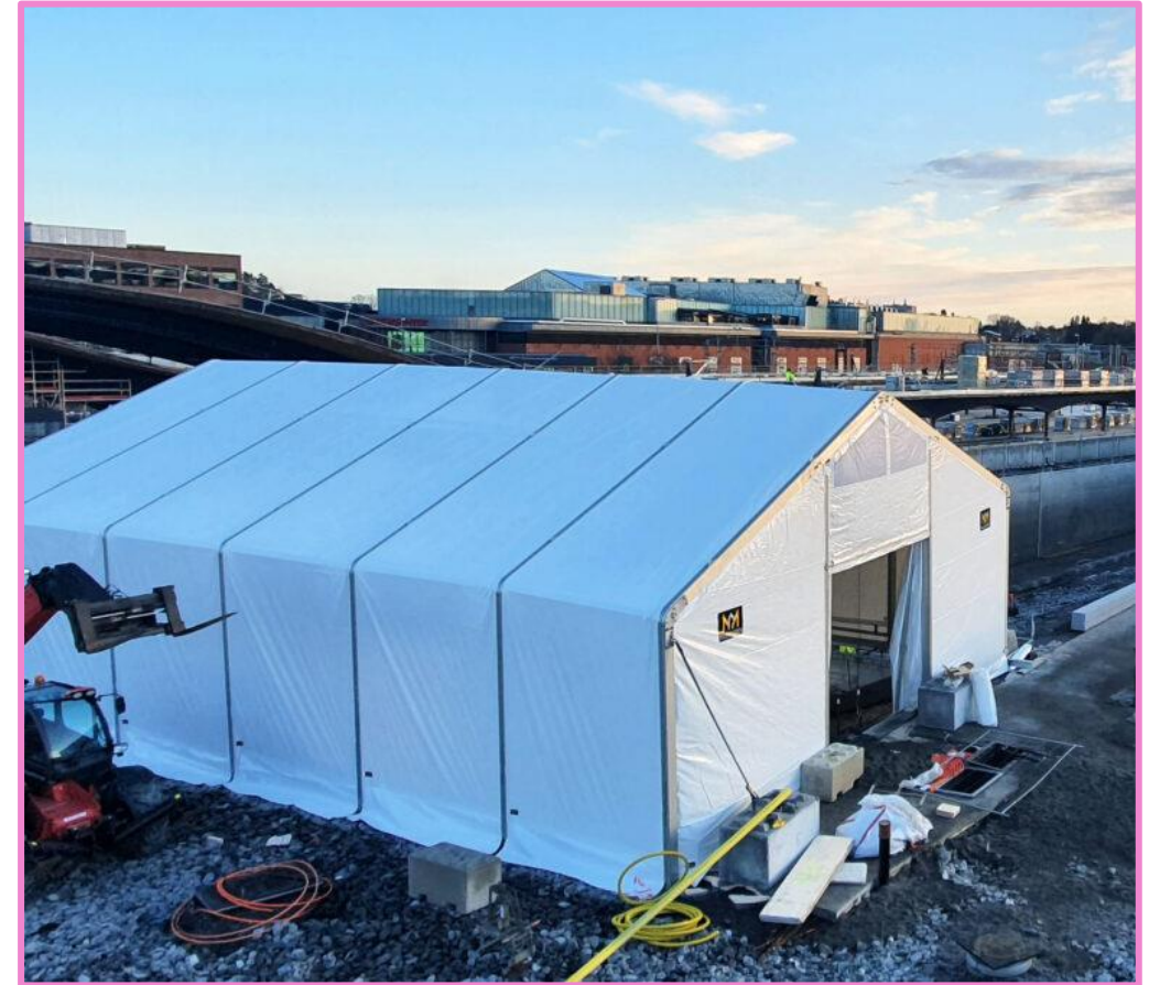
Example of an acoustic shelter tent, to protect from noise, dust and weather during excavation.
