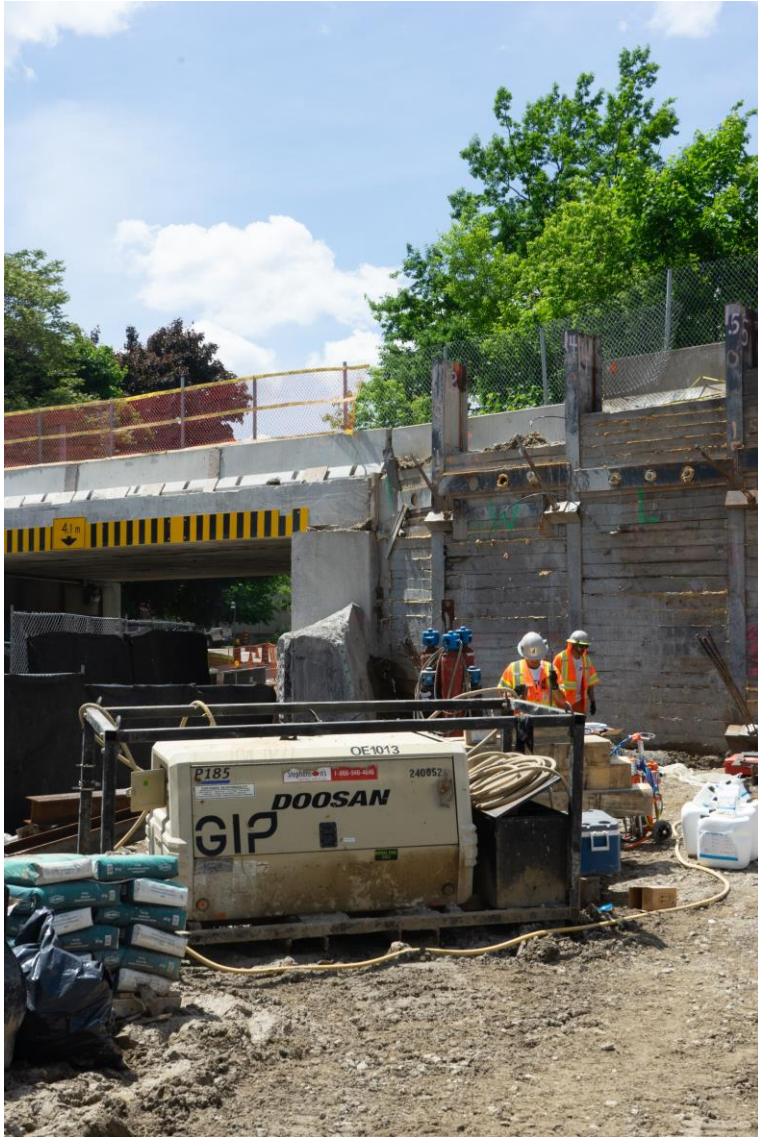
Lagging works and a part of the old abutment at Dundas St. E.
