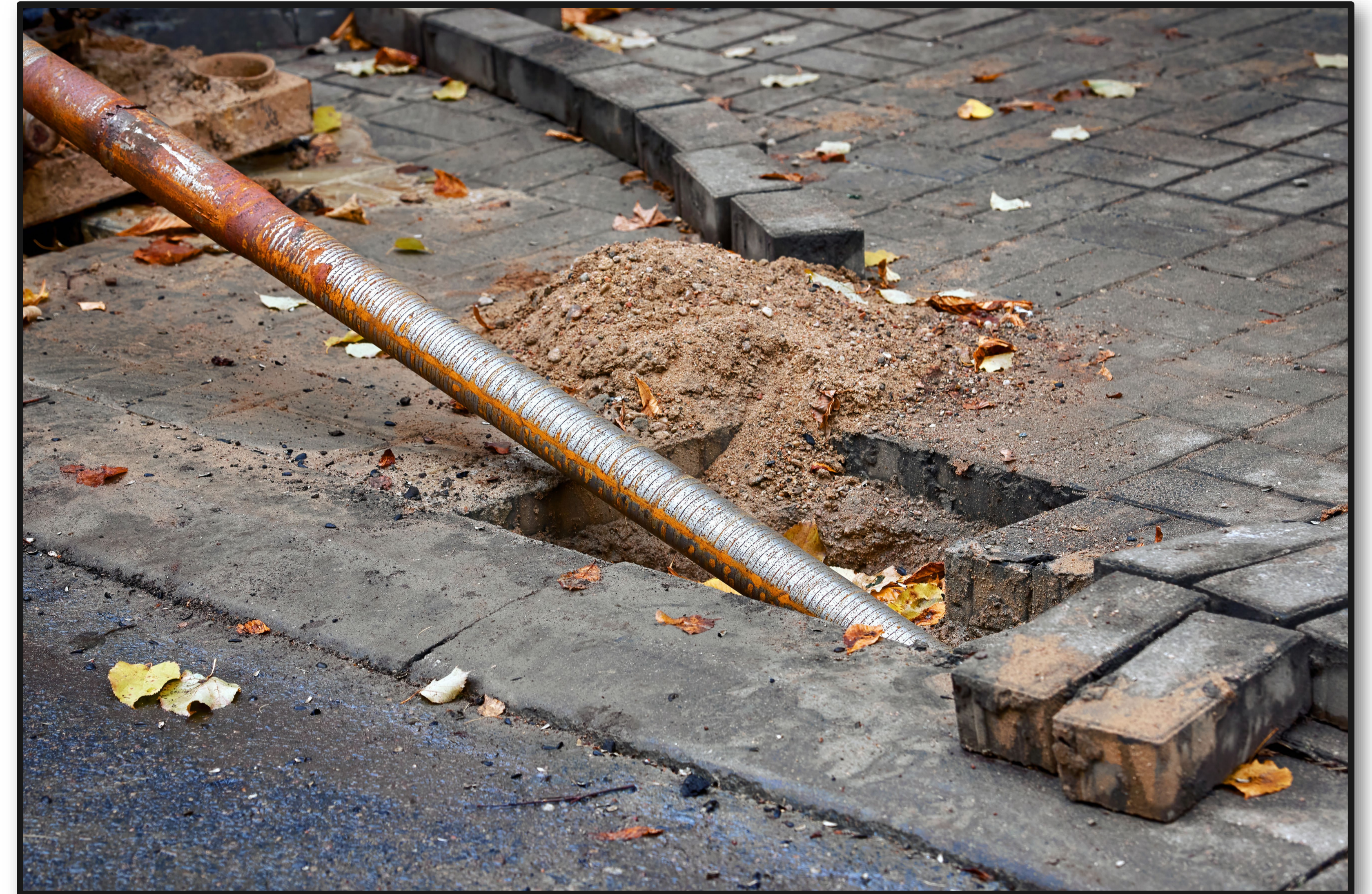
Directional drilling will be used to install cables under the laneway while minimizing disturbance to the surface (stock photo).
