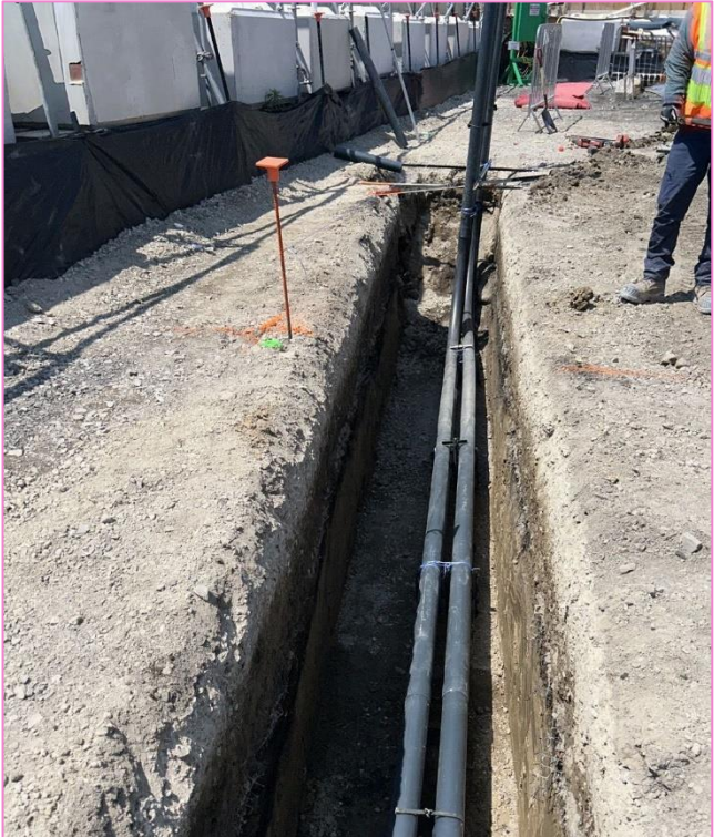
Site servicing - power distribution through the site.
