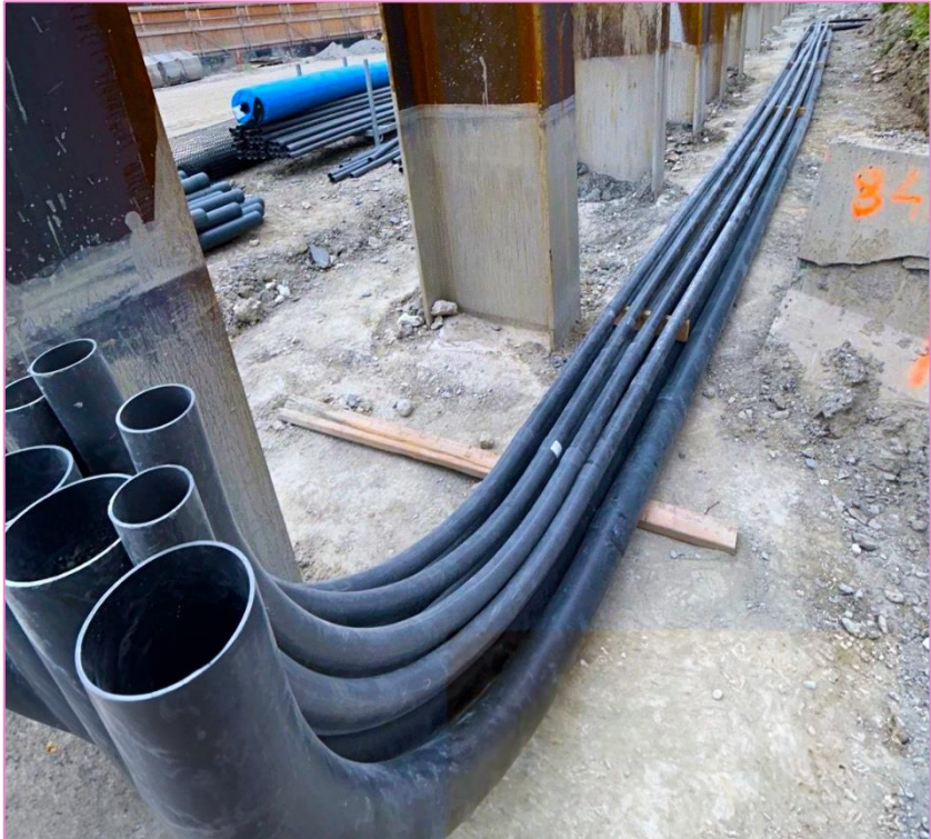
Site servicing - power distribution through the site.
