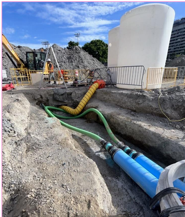
Pump and tank connection.
