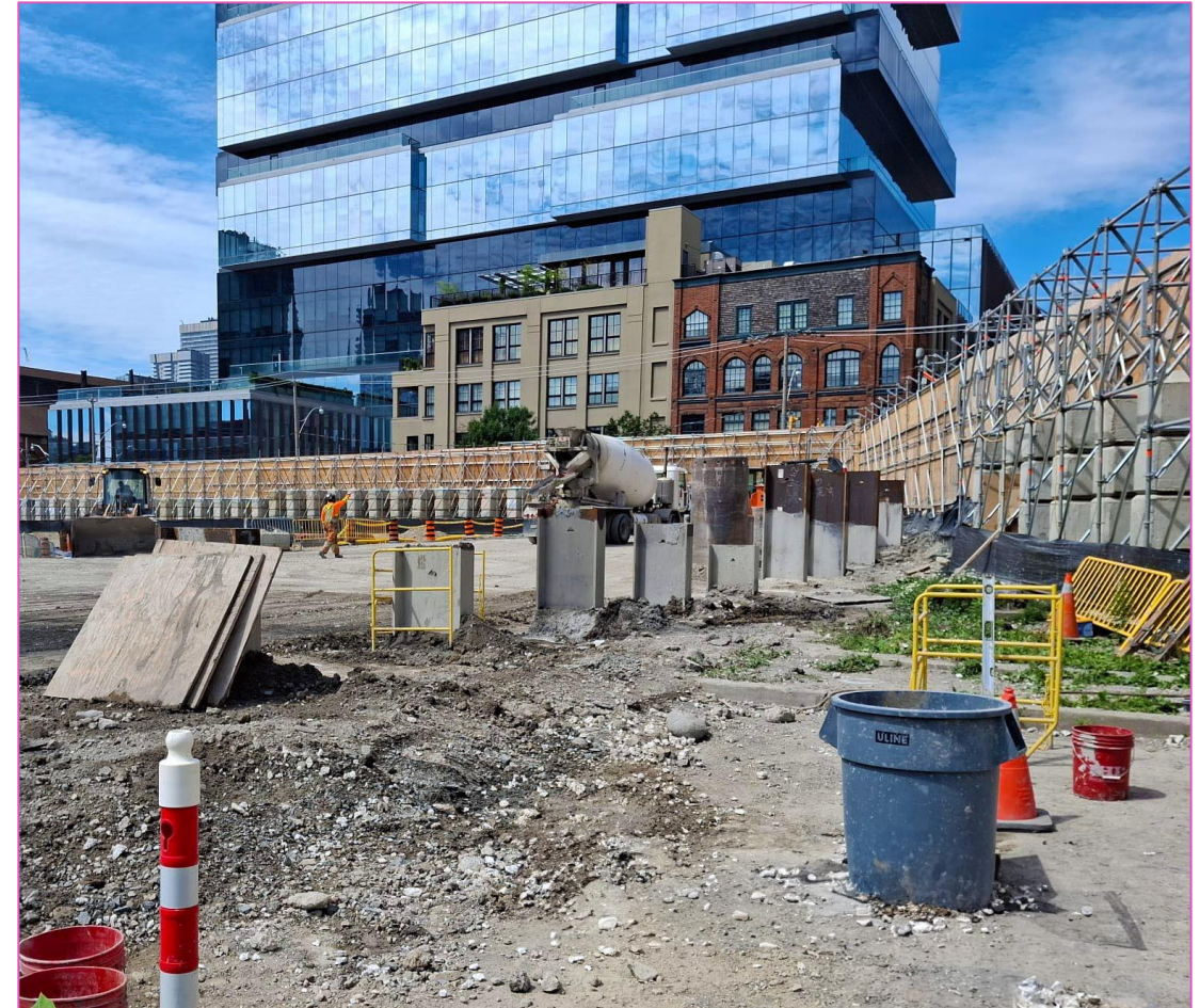
King piles and filler piles along the north shaft wall of the north site
