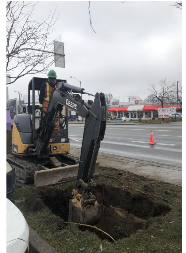
Excavators (or diggers) are used to dig holes or carry heavy equipment around the construction site.
