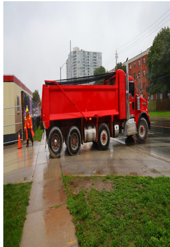
Dump trucks are used to remove the dirt from tunnelling or building underground stations.
