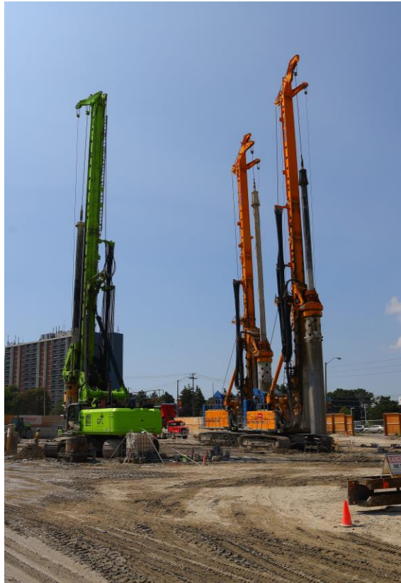
Pile drivers are used to put large poles into the ground that can support the new stations and buildings for LRTs and subways.
