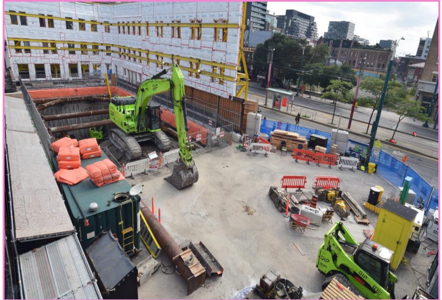
View of ongoing excavation work at the future north station site in late August 2024.
