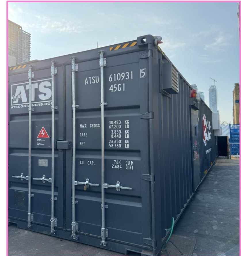
View of the substation power installed
