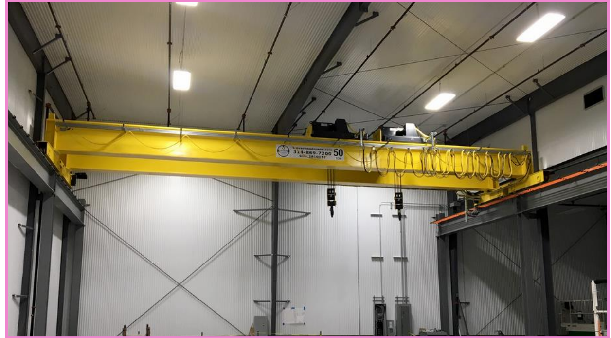
Example of an overhead crane; a mobile crane to help hoisting operations within the long-term acoustic shelter.
