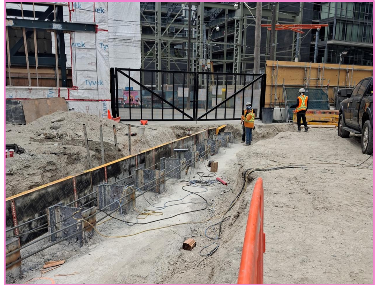
Crews prepare to install capping beams on piles, by connect horizontal rebar to the king piles.
