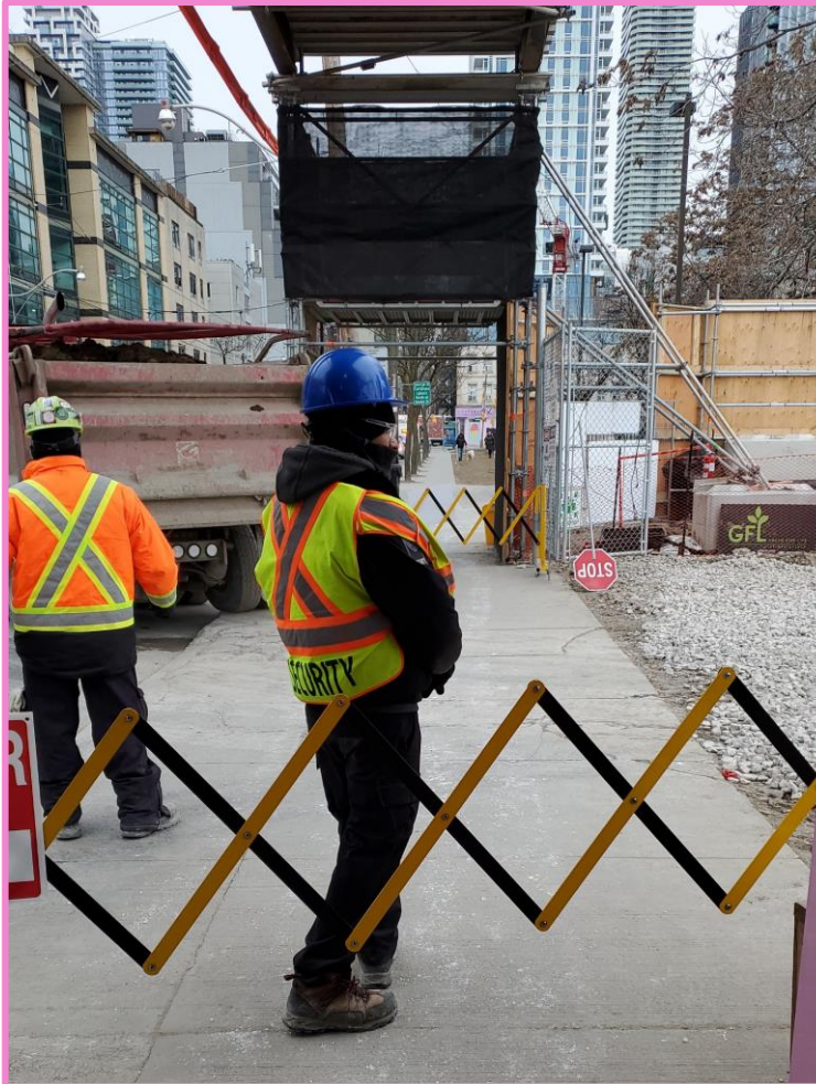
Accordion safety gates to allow trucks to enter and exit sites, protecting pedestrian safety.
