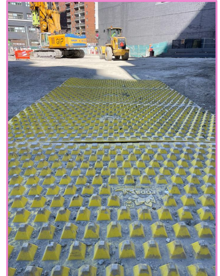
Wheel cleaning shaker mat, to ensure trucks do not bring mud and soil into city streets. Paving is also underway on site.
