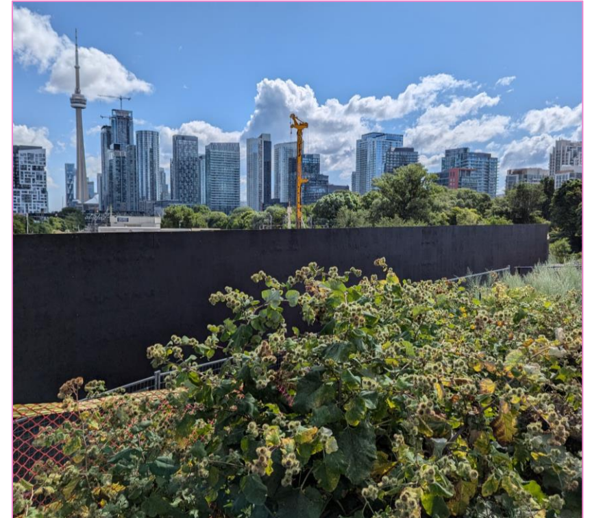
Right: Protective hoarding in front of the site, against the city backdrop.
