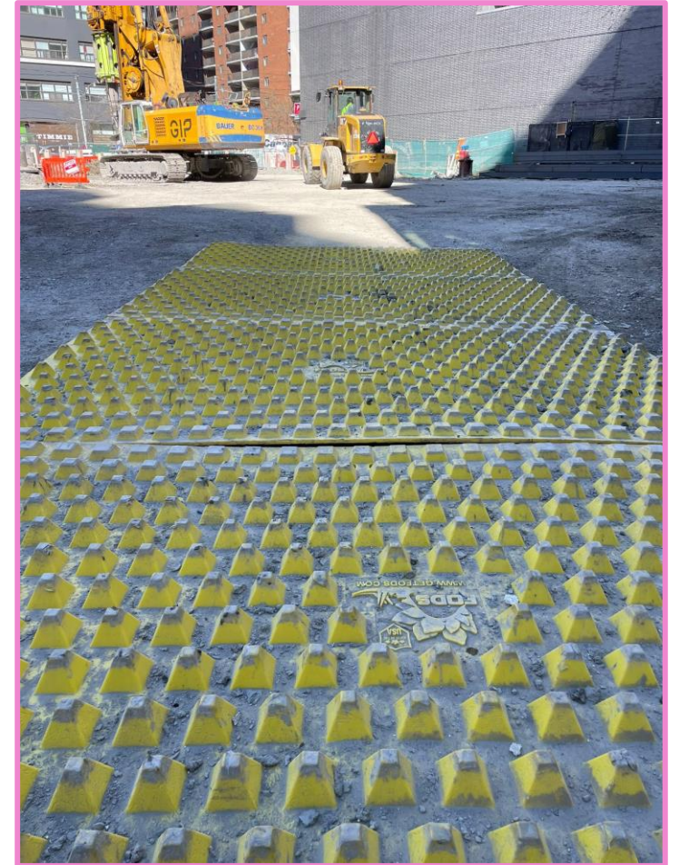
Wheel cleaning shaker mat, to ensure trucks do not bring mud and soil into city streets.
