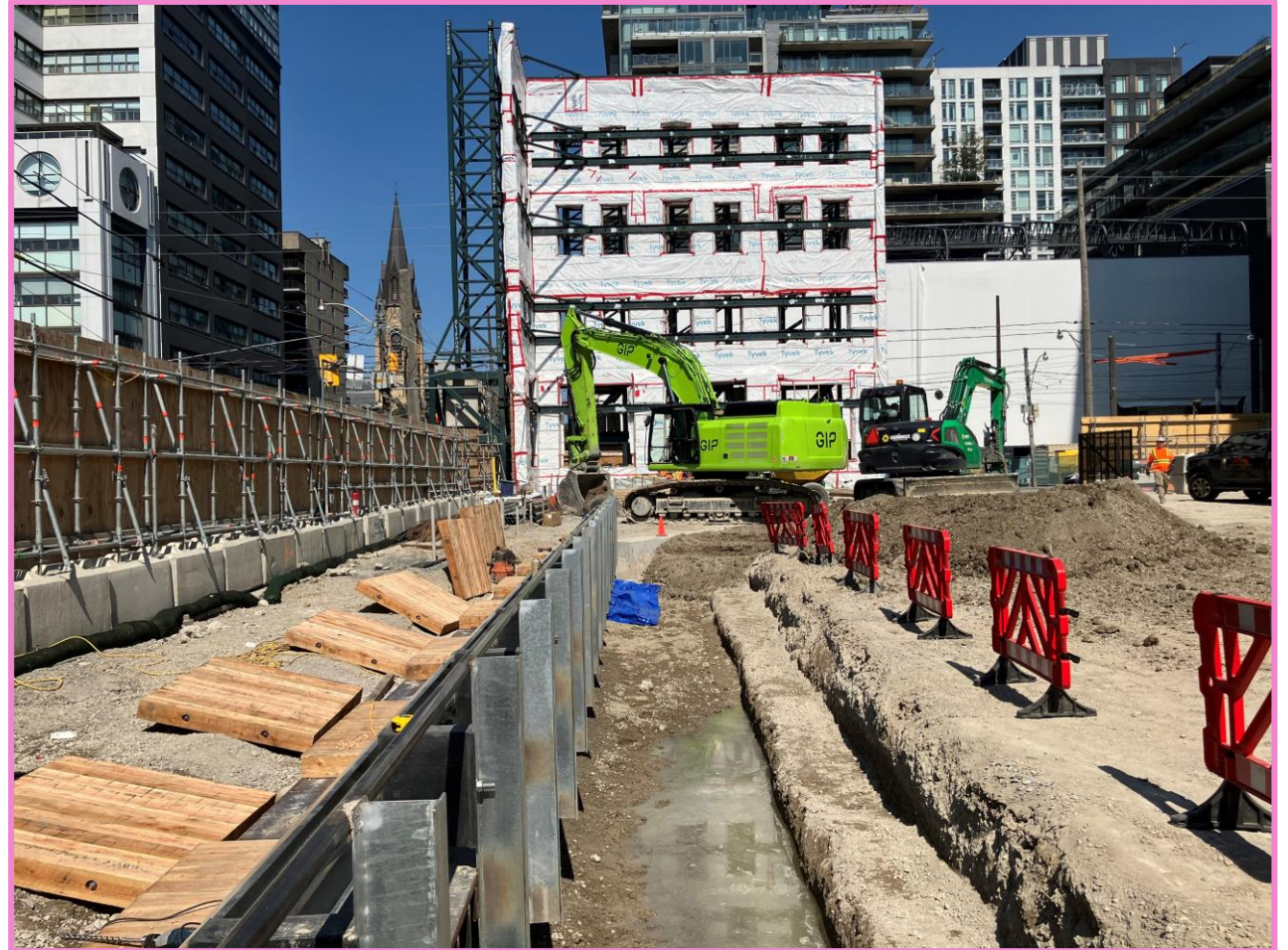
Crews complete capping beams on piles, by connect horizontal rebar to the king piles.
