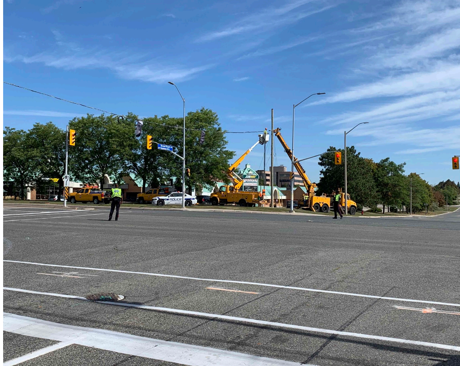
Temporary Traffic Signals
