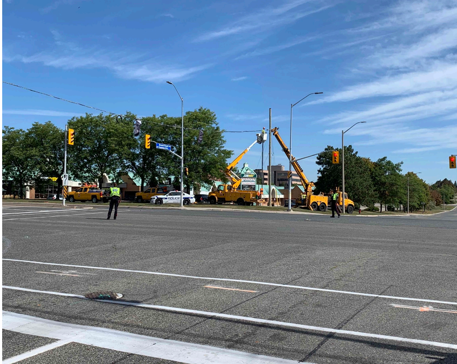
Temporary Traffic Signals
