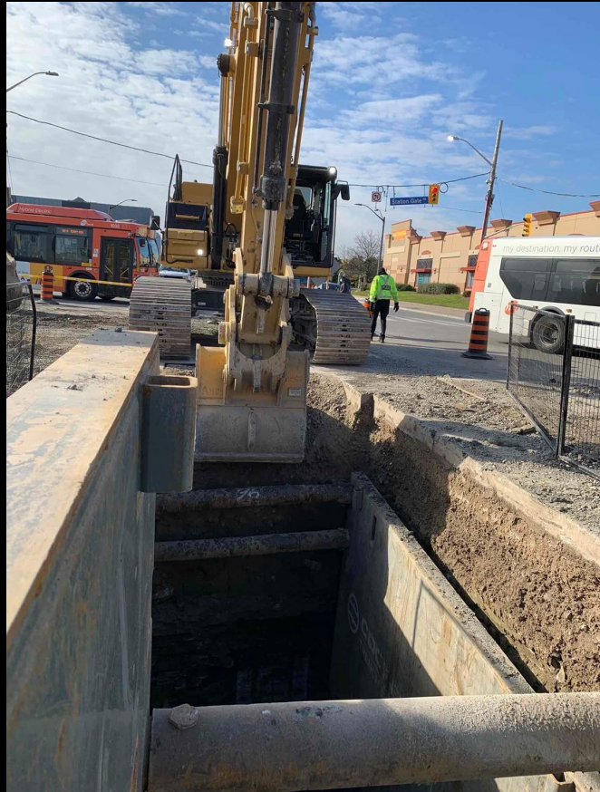
Sanitary Installations along Rathburn Road in Mississauga Centre
