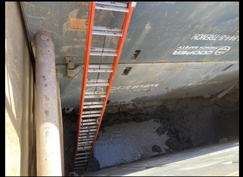
Sanitary Installations – Mississauga Centre
