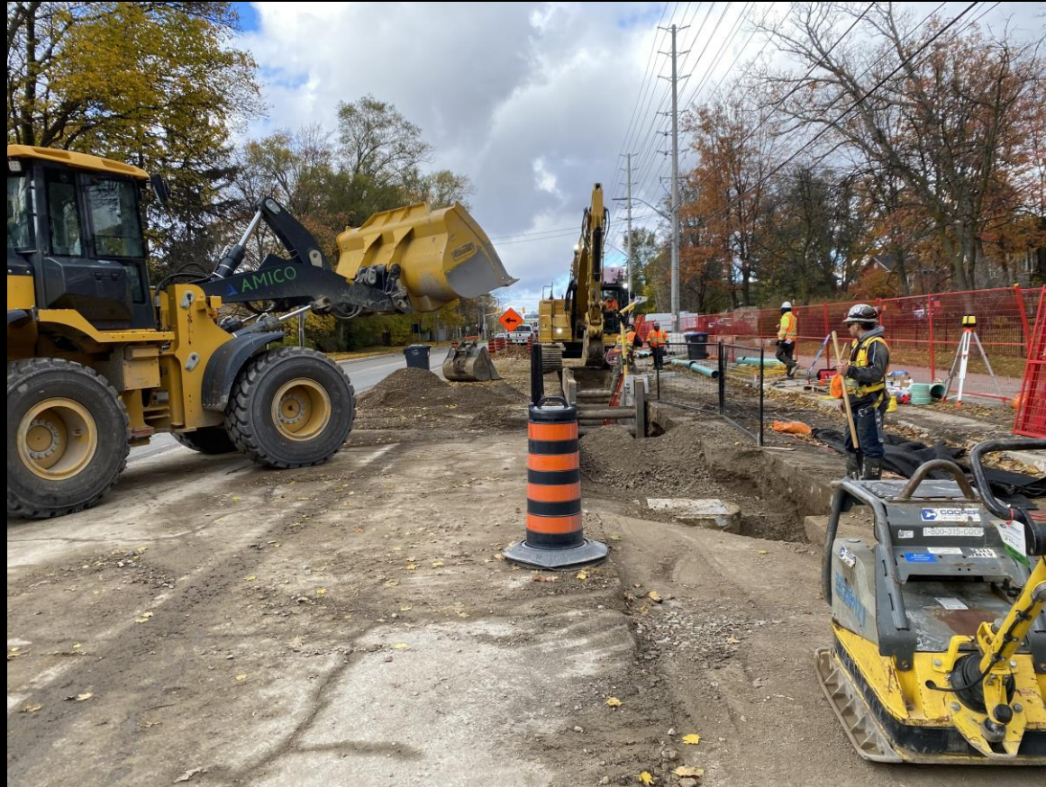
Sanitary Installations – Mississauga South
