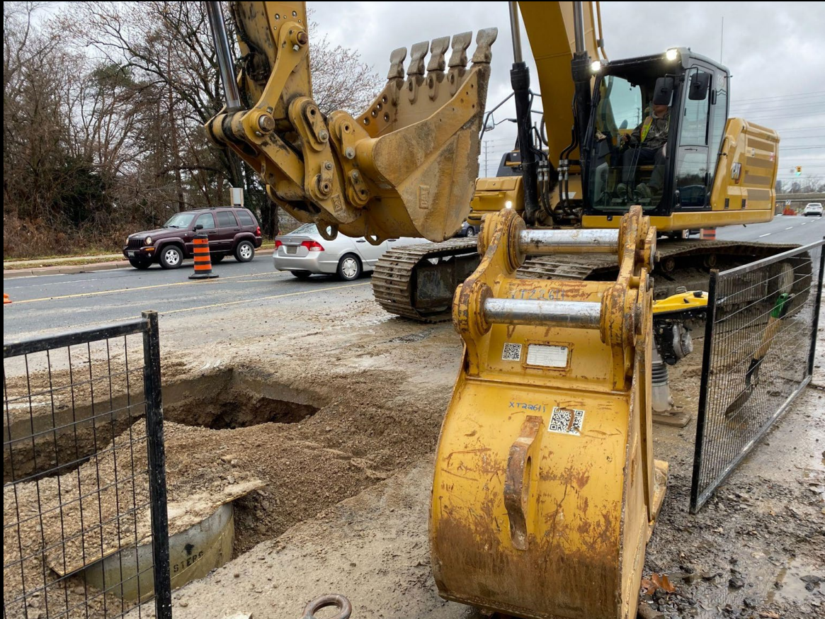
Sanitary Installations - Mississauga South
