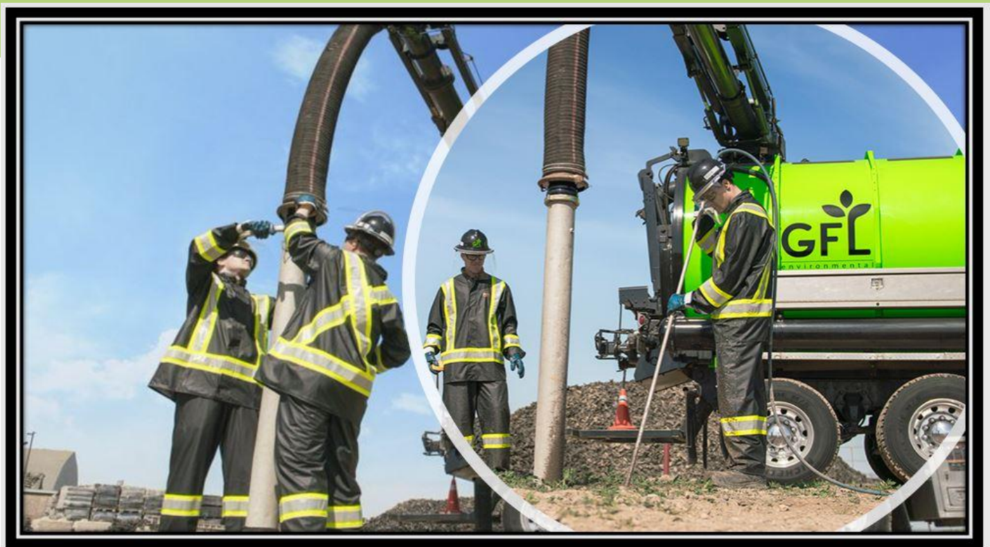
GFL crew using a hydrovac truck to expose intricate utility infrastructure as found in the Union Station Rail Corridor - East (photo courtesy of GFL)
