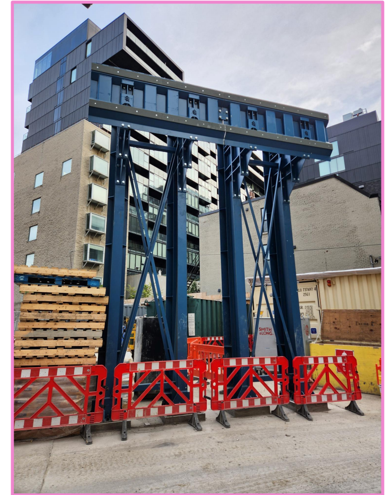
Structural support for self-dumping bin to be installed, on top of dump trucks.
