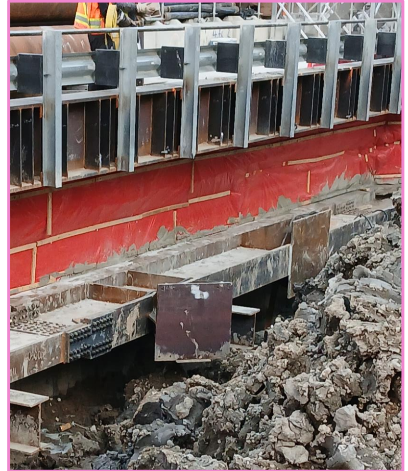
Crews complete capping beams on piles, by connecting horizontal rebar to the king piles.
