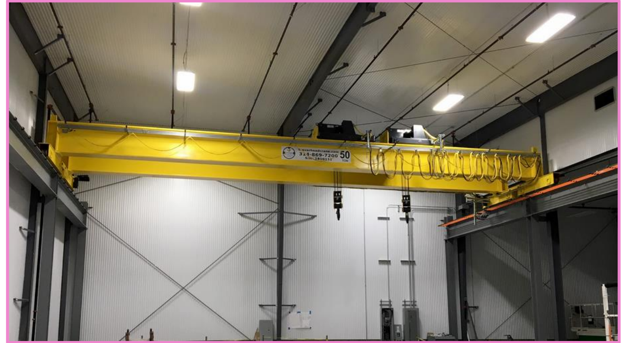
Example of an overhead crane to help hoisting operations within the long-term acoustic shelter.
