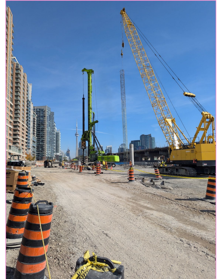
Piling to reinforce the ground to ensure structural integrity for excavation and foundations.
