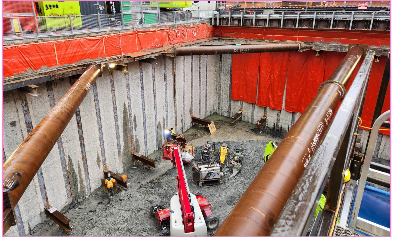
Example of installation of struts and walers (beams protruding on the left) while excavators dig down, to a future Ontario Line station.
