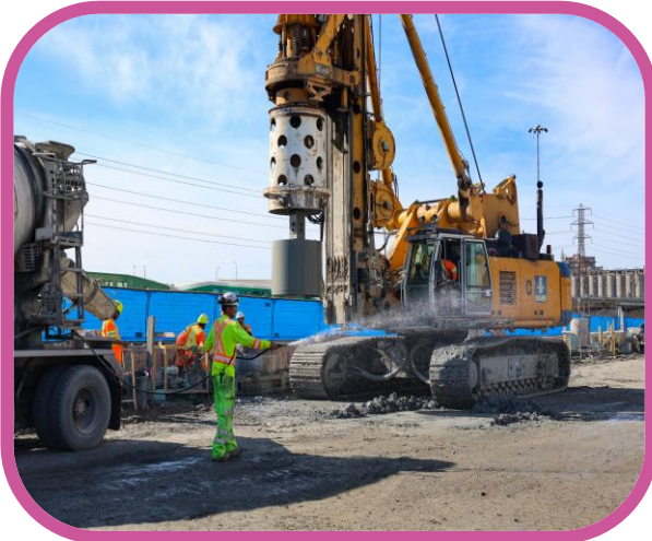
Water misting spoils
