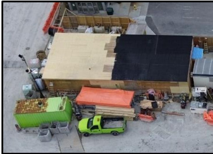
Enclosure around water treatment plant:
