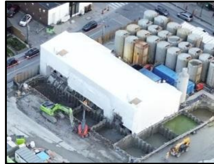
Enclosure around slurry plant:
