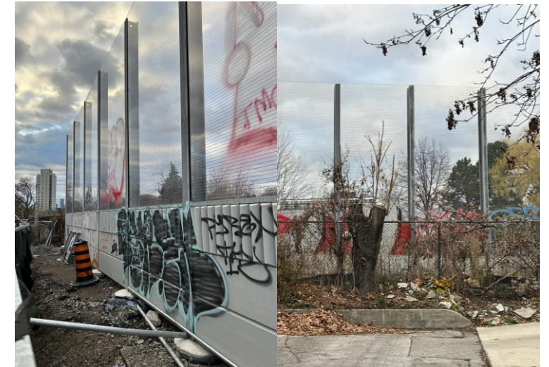
Graffiti on noise barriers at grade
