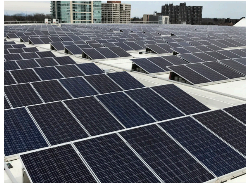
Clarkson GO Station. On top of the 1,500-space, five-storey parking structure, the roof is entirely covered with solar panels.
