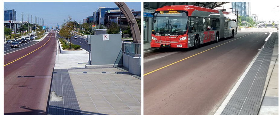
Figure 5-5: Tactile walking surface indicator at edge, damage observed (left) and tactile walking surface indicator set back 125 mm (right)
