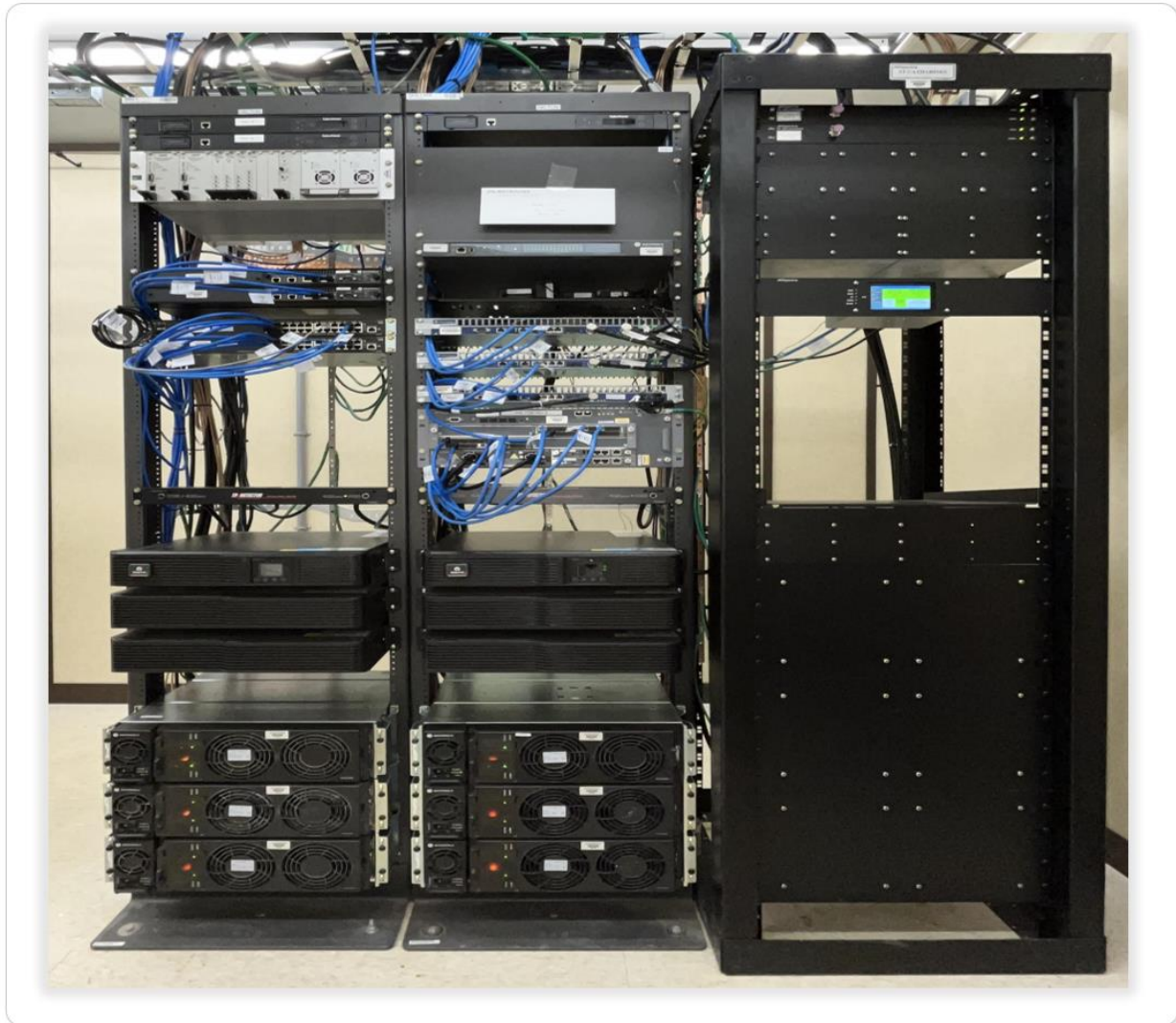
Figure 11: Radio Systems Rack
