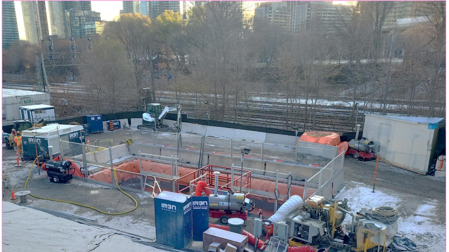
The excavated shaft at Ordnance Park which will lead to a small integrated exit building in the park.
