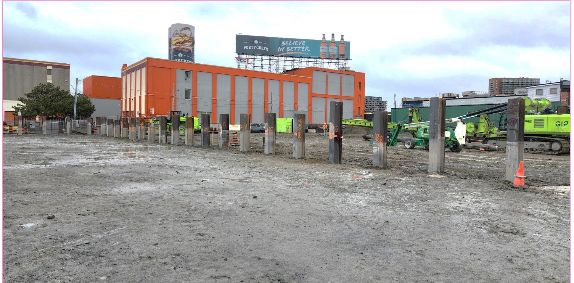
Future station building support piles between Jefferson and Atlantic Avenue, looking northwest.
