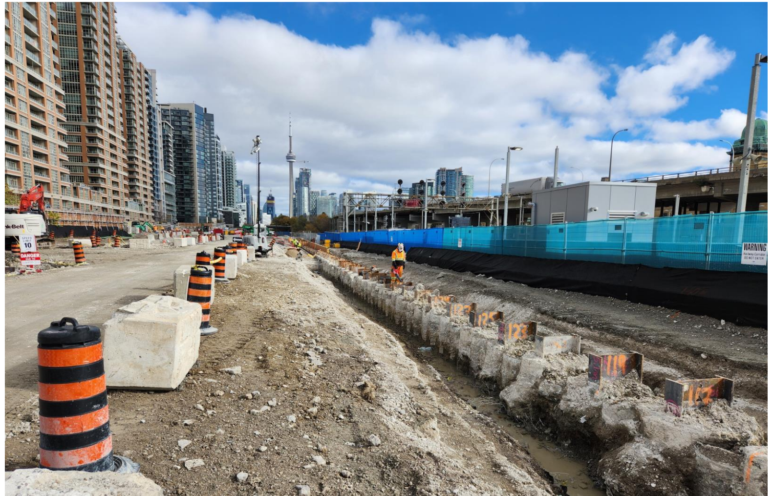
Piling to reinforce the ground to ensure structural integrity for excavation and foundations, looking east.
