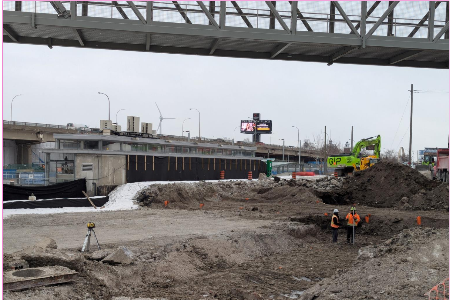
Looking southwest at the TPSS location, beneath the pedestrian bridge.
