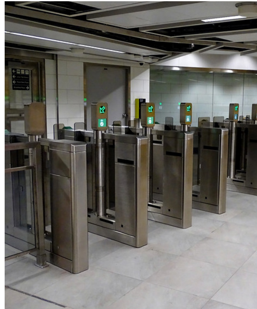
Figure 10: Typical Fare Gate - TTC Union Station
