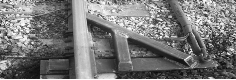
Figure 10. Rail grip used to anchor rail to track structure
