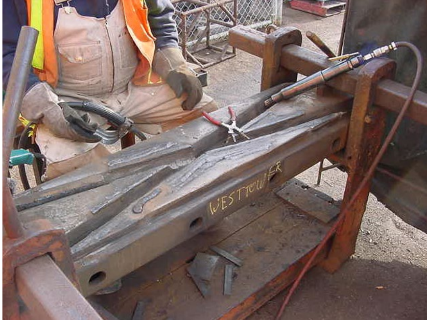
Figure 14-6: Diamond Crossing Insert Being Repaired in a Strongback Jig Courtesy CN Training
