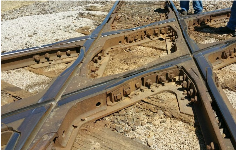
Figure 6-49: RBM Railroad Crossing Diamond
