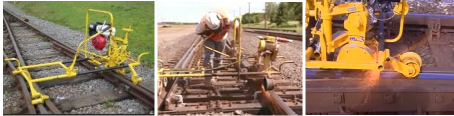
Figure 5-6: Switch Grinders Courtesy IRS, Pinterest, and CN Training
