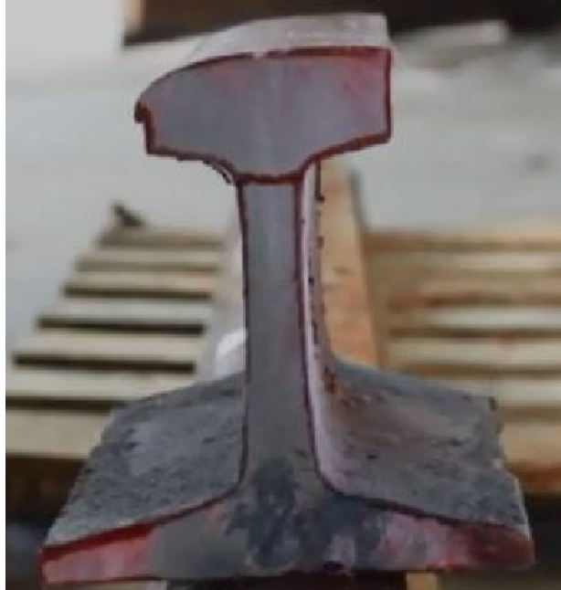
Figure 9-2: DP Tested Rail with a Horizontal Split Web Defect in the Head-Web Intersection
