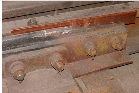
Figure 7-8: Photo of a Copper Backing Plate Between Switch Point and Stock Rail Courtesy CN Training
