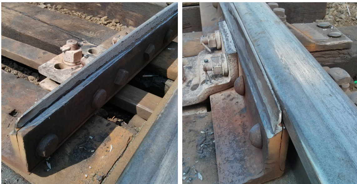
Figure 6-14: Examples of Knife Switch Point Grinding after Weld Repair Courtesy CN Training
