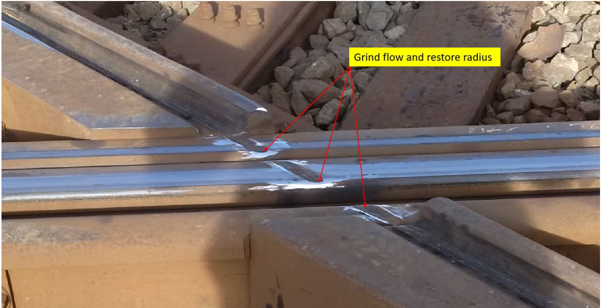
Figure 6-28: Grinding Areas on a Flange Bearing Railroad Crossing
