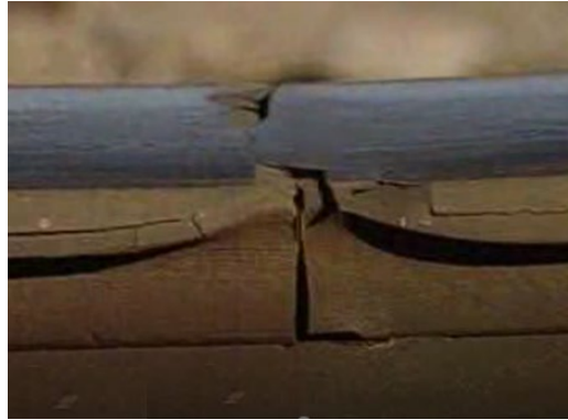
Figure 6-15: Overflow at Joint
