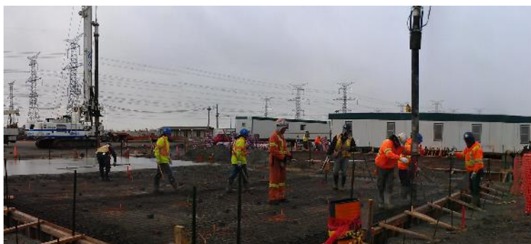
Auxiliary installations YYSSE
